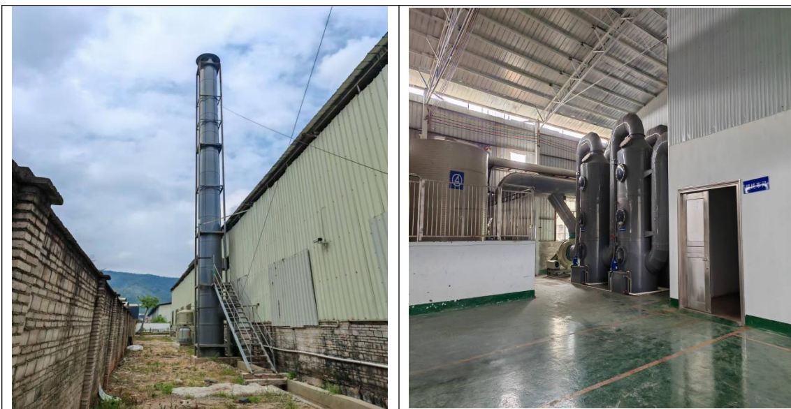
精炼线碱性废气排放口DA012
